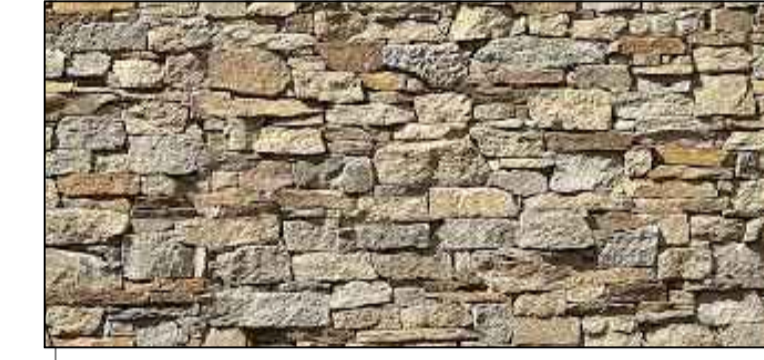
VIEW TO BOUNDARY WALL WITH NATURAL STONE BOTH SIDES - WALL WITH RECESSED JOINT
